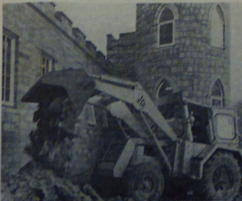
Preliminary work already under way on the new wing to the Saint Hill Castle.
